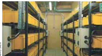
Local battery application.
